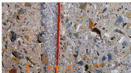
Secondary sprayed or cast concrete lining TamSeal 800 – 1 st coat orange, 2 nd coat grey Regulating layer such as TamCrete TopShot Primary sprayed concrete lining
